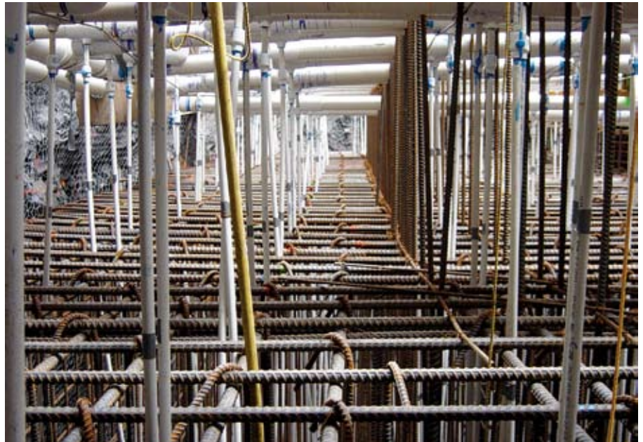
Fig. 1: PVC cooling pipes connected to main supply headers circulate cooling water to control the temperature of the concrete as it cures
