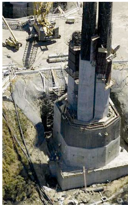
Fig. 5: One of two 19 x 19 x 10 m (63 x 63 x 33 ft) footing blocks for the self-anchored suspension structure
