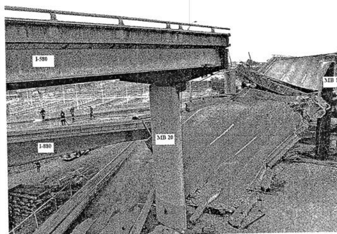
Two spans of I-580 collapsed onto the I-880 connector ramp directly below.
